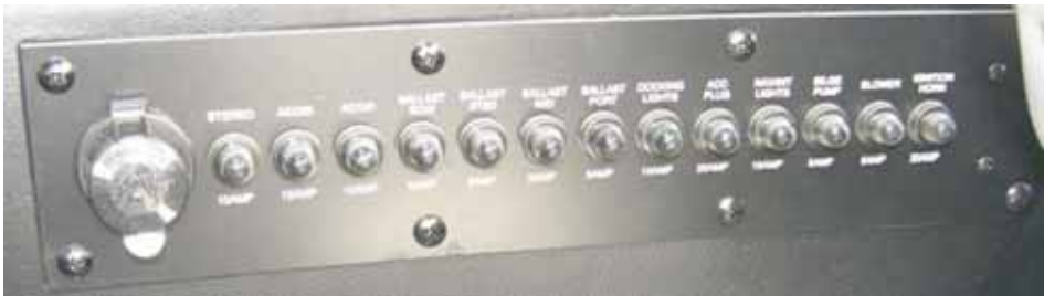
Figure 2-4. Circuit Breaker Panels
