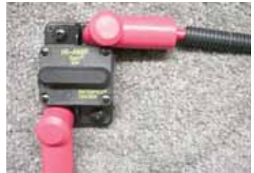
Figure 4-4. Main Circuit Breaker
